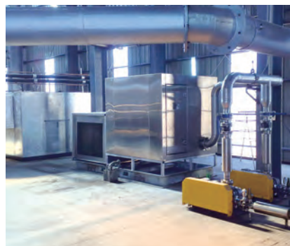
Air Chiller and Blowers
